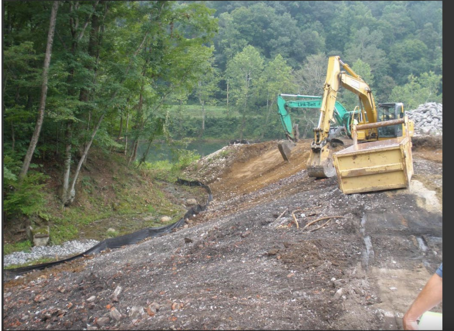
ERS excavate lead-contaminated soils along the western bank of the western area of the Site. ERS placed silt fence and rip-rap along the runoff area.
