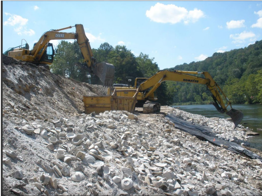
ERRS utilize excavators with mechanical thumbs, along with a rock box, to place rip-rap along the river's edge
