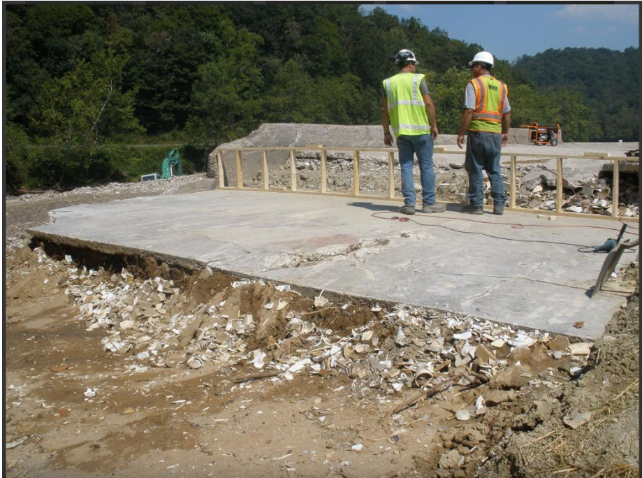
ERRS prepare to use cement to encapsulate exposed materials in the western area of the site
