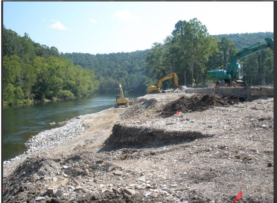
START conducts XRF screening for lead concentrations that remain in the site materials
